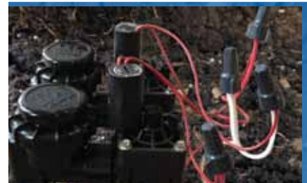
irrigation and sprinkler systems
